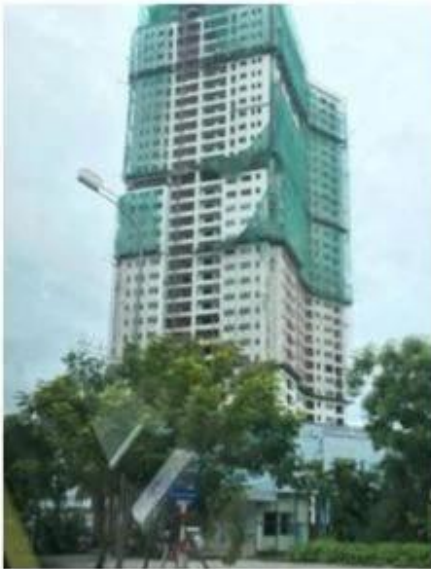
Blooming Tower I Vietnam 16MM Clear IGU 6000m2, 55.4 Clear ESG VSG PVB 4000m2
