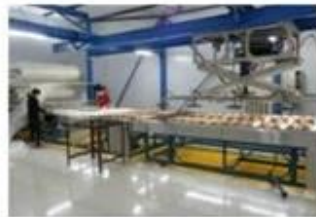
合片室设备 Clean Room Equipment
