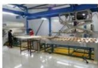
合片室设备 Clean Room Equipment
