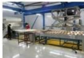
合片室设备 Clean Room Equipment
