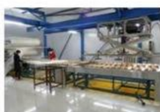
合片室设备 Clean Room Equipment
