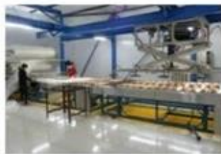
合片室设备 Clean Room Equipment
